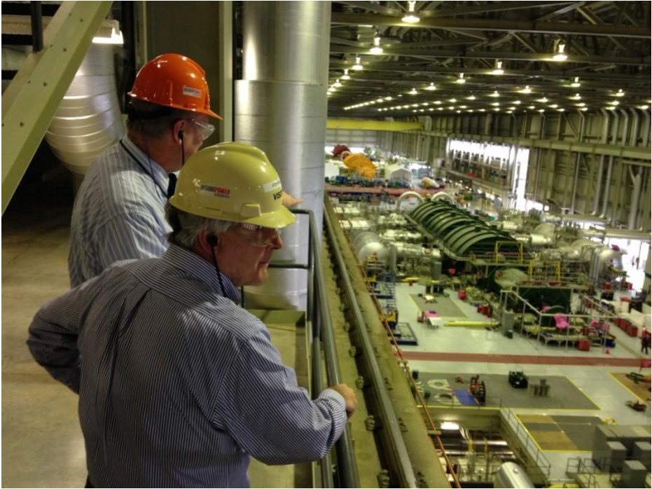
Former NRC Chairman Stephen Burns (right) stands with Brian Duncan, retired Senior Vice President at the Darlington nuclear power plant in Ontario, Canada, examining the turbine building during a tour of the plant
