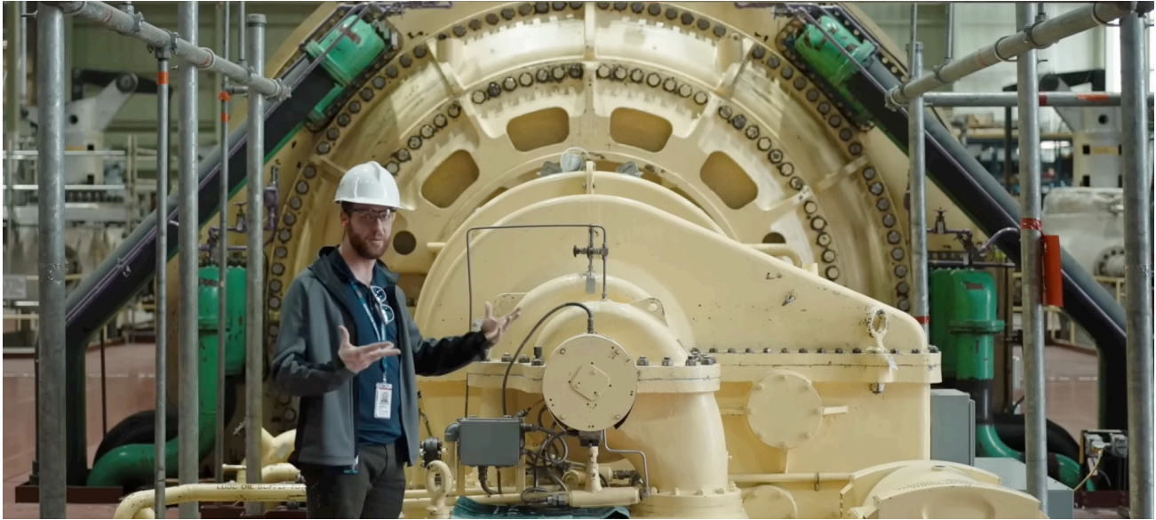
Authorized Nuclear Operator Dan Campbell stands in front of steam turbine at Bruce Nuclear Generating Station Unit 4, Decouple Media
